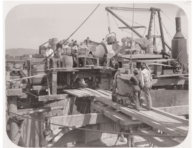
54. CEN CAL RY. Placing Concrete in Pivot Pier, Newark St. Draw Aug 21, 1908
